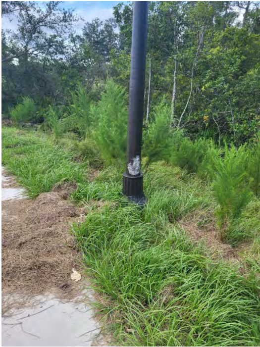
Location 16: Street light pole damage.
