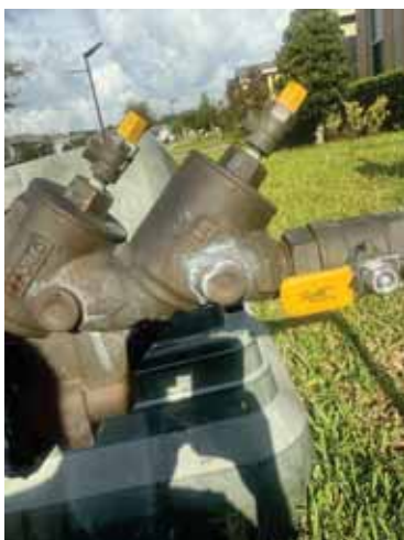
Original backflow cracked body
