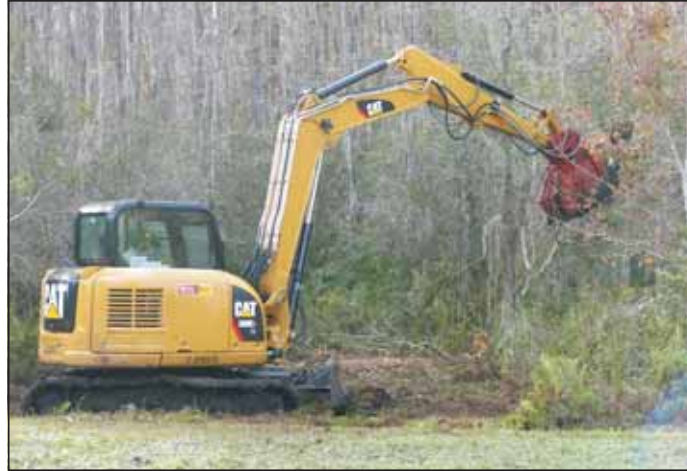
This excavator equipped with a mulching attachment did most of the work in clearing the wetland buffer zone, as shown in photos on page 11 at right.
