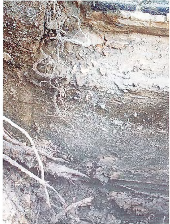
Tree roots in area where skimmer had to be replaced.
