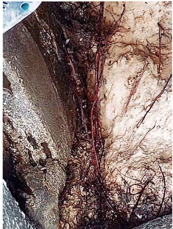
Tree roots in area where skimmer had to be replaced.
