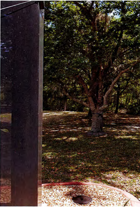
Tree roots encroaching on lanai and pool area.
