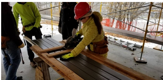
A student cutting materials for the park shelter their class is building.
