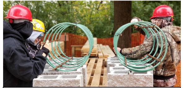
Students in the Building Construction 2 class, part of the ACE Academy, working on a new park shelter at Sunset Park in Kimberly, Wis.
