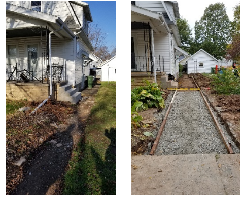
The sidewalk along the house before and during the construction work being done by Kimberly students.
