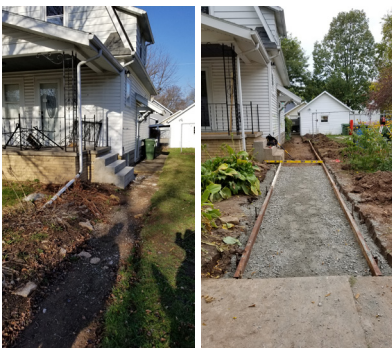
The sidewalk along the house before and during the construction work being done by Kimberly students.
