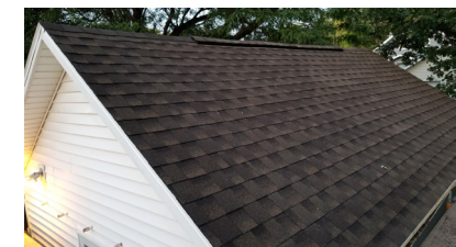
The garage before, during and after a new roof was installed by Kimberly High School students.
