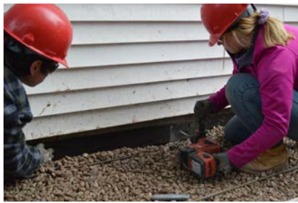
Spencer Stevens and Hannah Gegare working on the concrete form for a new sidewalk during their BC2 Class.
